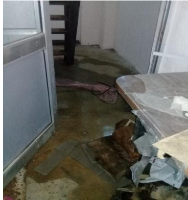
Rain water leakage
