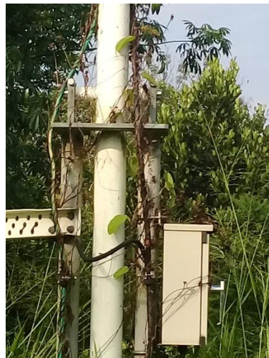
AWS System located at Wagolla (2019.03.15)
