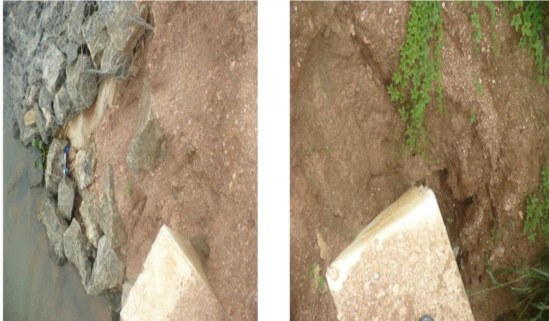
Guiding Wall and tank bund not constructed to stipulated standard on both sides of the spill gate (Photograph No. 7)
