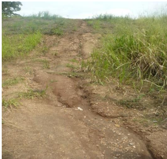
← Erosion of tank bund due to vehicle movement (Photograph No 03)
