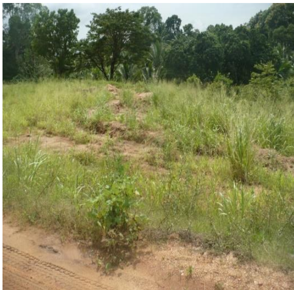
← Not applying turf on the tank bund (Photograph No 04)
