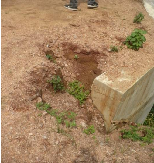
← Erosion of the Tank Bund at the instance of overflowing the Tank Photograph No 05
