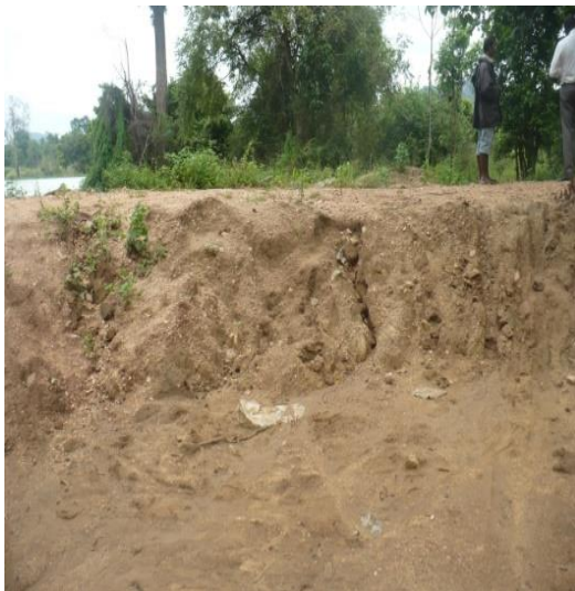
← Saddle Dam not constructed in stipulated standard (Photograph No 06)
