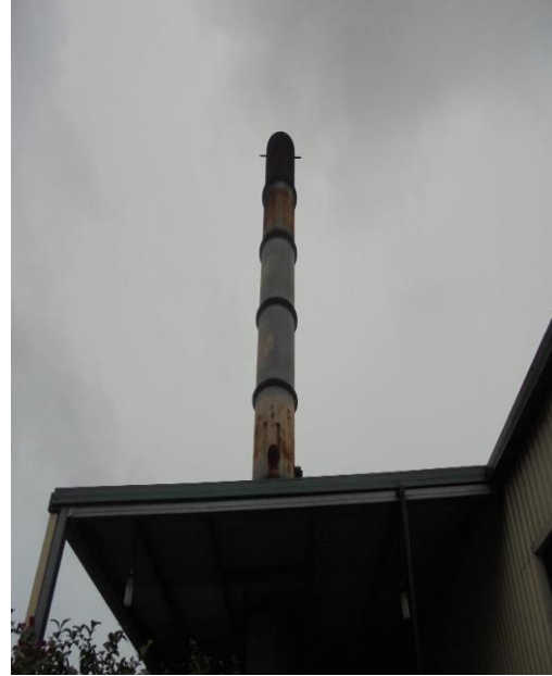
Photo- Chimney of the incinerator without top cover at the Polonnaruwa Hospital.
