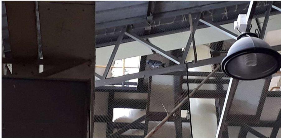
Figure No 01 - Pigeons staying inside the building of production section
