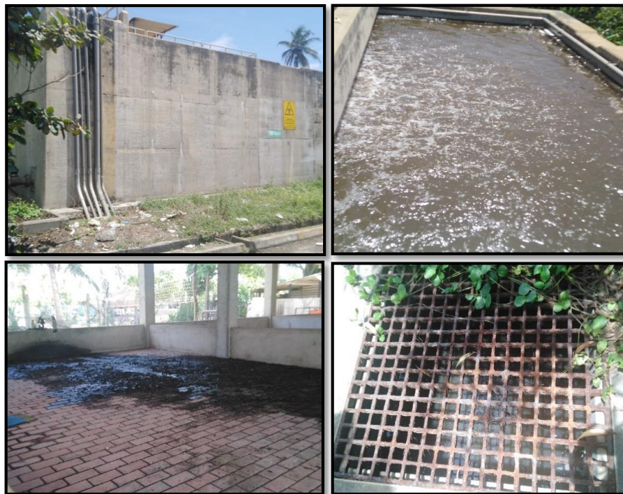
Figure - 01 Dikowita Port Wastewater Treatment Plant
