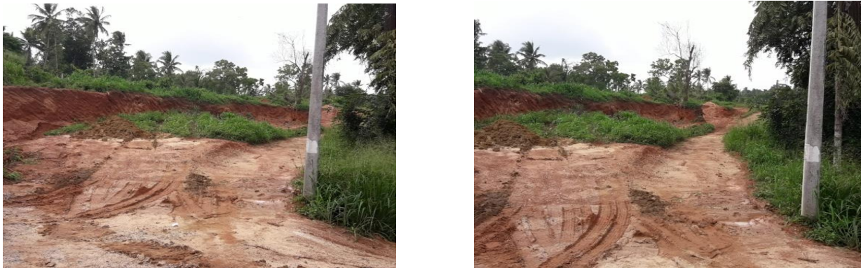
Figure 13 - How the environment near the Bogoda Tank was damaged
