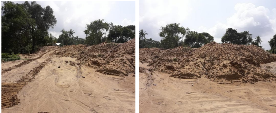
Figure 12 - A large amount of gravel soil around Bogoda tank
